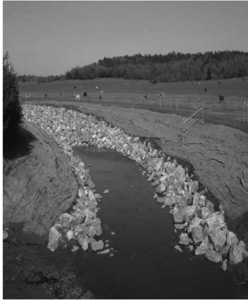
Figure 6. Grade Stabilization, Gracemont, Oklahoma
